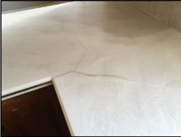
kitchen solid surface counter damaged
