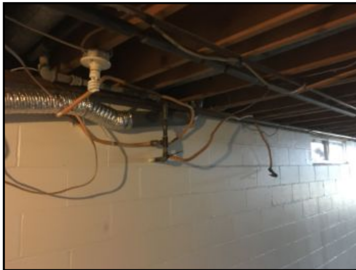
Flexible gas line needs to be terminated
