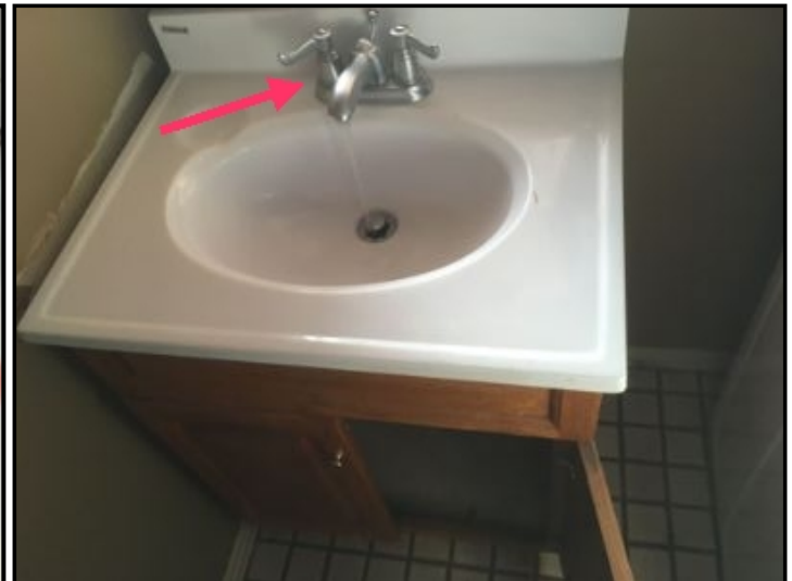
Aging fixtures in first floor 1/2 bath
