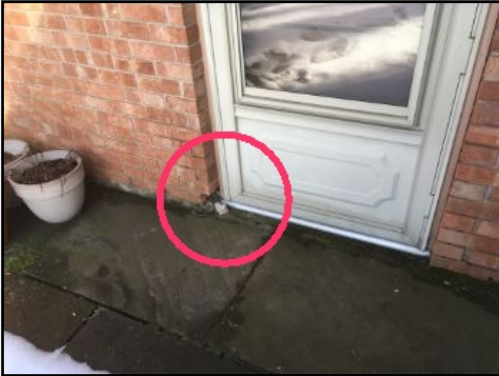
Minor brick deterioration around rear entry door due to roof water splash
