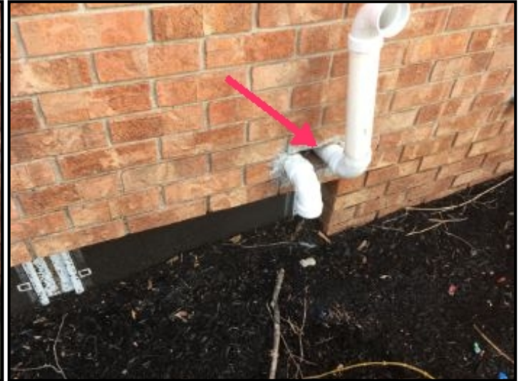
poor retrofit of furnace venting- brick needs sealing
