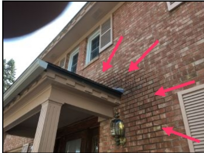
Lack of upper roof gutters causing brick deterioration
