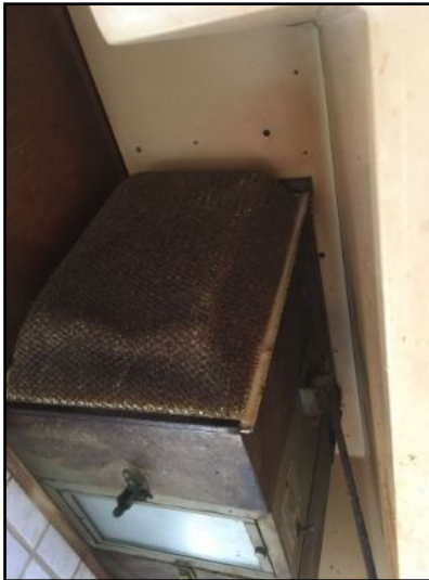
Filter and hood system over stove very marginal
