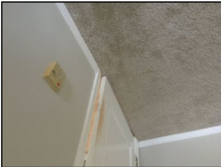
dog damage to master bedroom door
