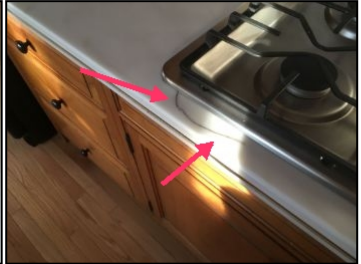
Kitchen counter solid surface damaged at stove
