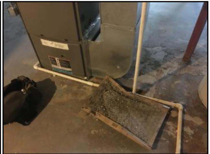
furnace presently working without filter-new filter needed.
