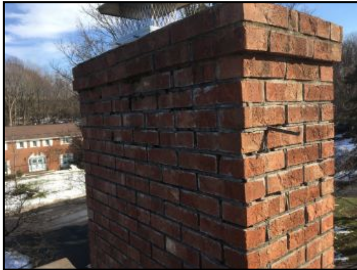
Chimney crown needs moderate amount of work-repointing and water sealing
