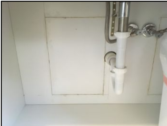
plumbing pipes on outside wall-questionable-possible repairs previously
