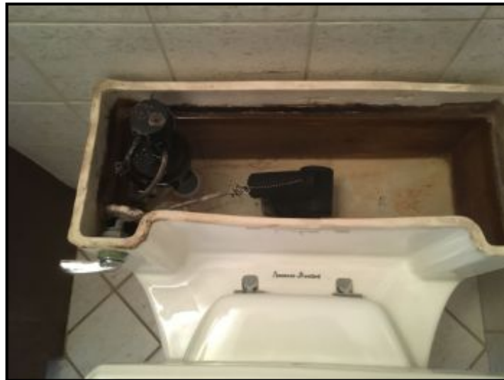
toilet in 1/2 bath marginal-toilet tank valve aging
