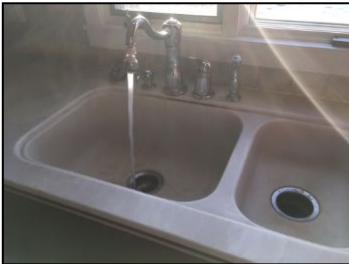
Aging sink and faucet in kitchen-faucet h
