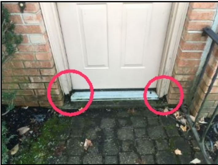
Breezeway entry door on front damaged due to roof water splash-needs replacing
