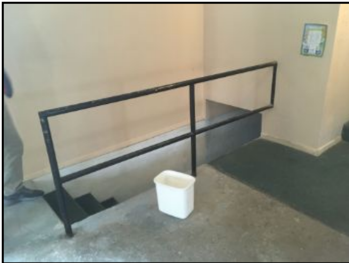
garage safety rail not safe due to wide spacing
