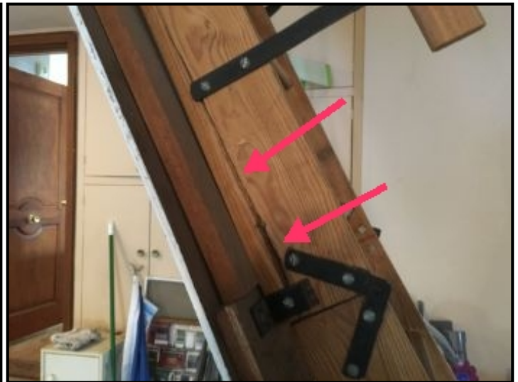
roof ladder damaged -needs repairs for safety
