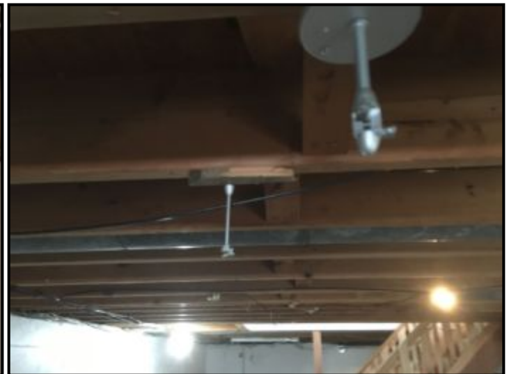
Misc. lighting in basement need terminating or replacing
