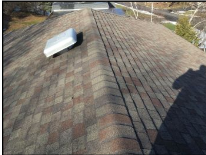
Roof ventilation is modest lacking ridge vent
