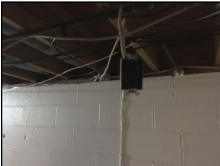
loose wiring and exposed outlets should be properly secured or eliminated
