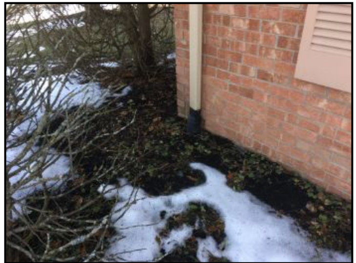
underground downspout leaders questionable- don't resurface-need to be corrected
