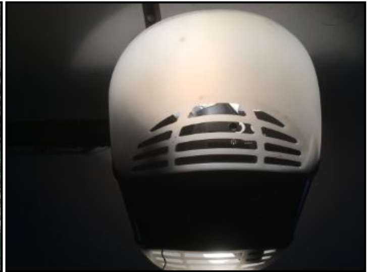
garage door operator needs to have downward pressure reduced for safety
