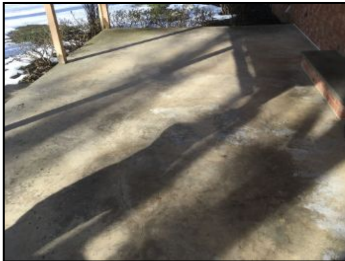
patio slab has spider cracking but found in reasonable condition
