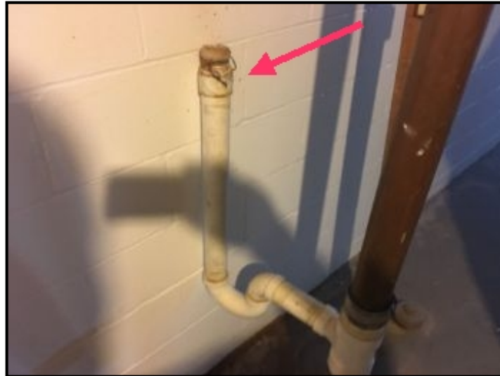
unused laundry drain on basement needs to be terminated
