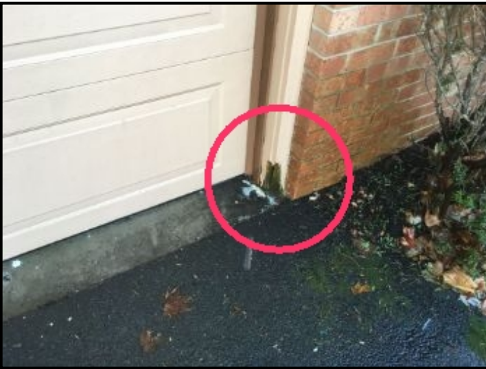
Overhead garage door jamb and trim heavily decayed at base due to roof water splash
